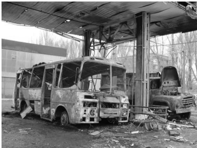
Figure. Damage to vehicles and building structures as a result of methane-air mixture explosion at the multifuel filling station
