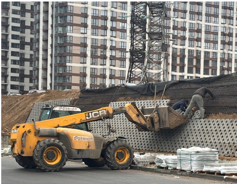
Fig. 3. Working from the bucket of the JCB telehandler in violation of health and work safety requirements
